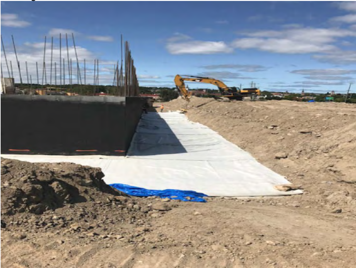
Building view to the north – installation of clay liner at foundation walls
