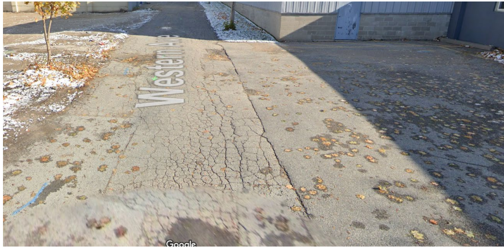
Western Avenue – PCI 36
