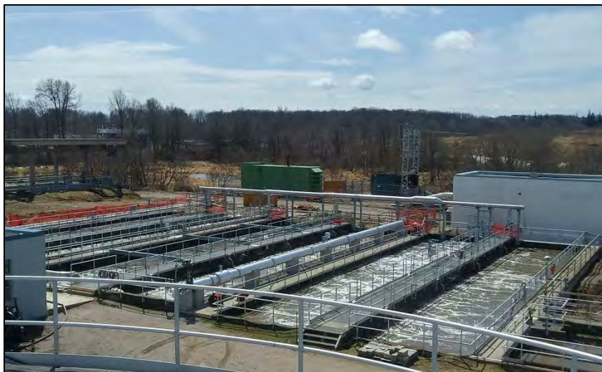
Figure 5 – Six-Pass Aeration Channels
