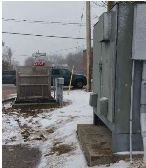
Figure 25 – Pumping Station No. 19
