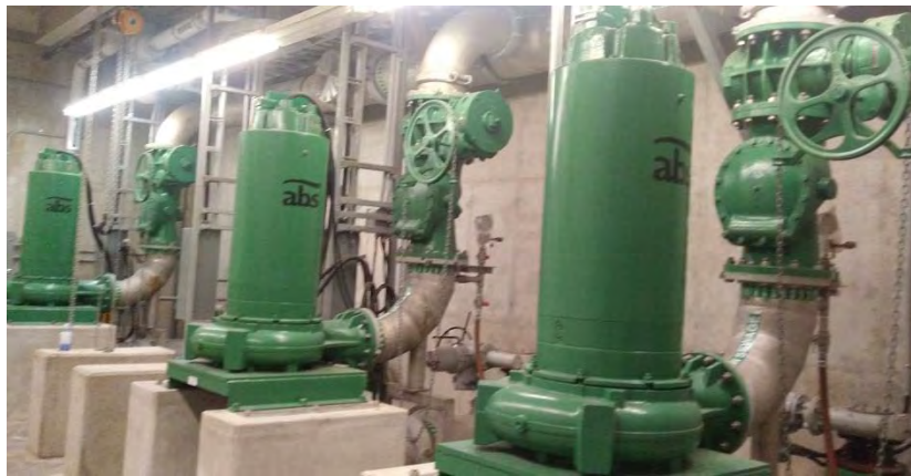
Figure 30 – Pumping Station No. 23
