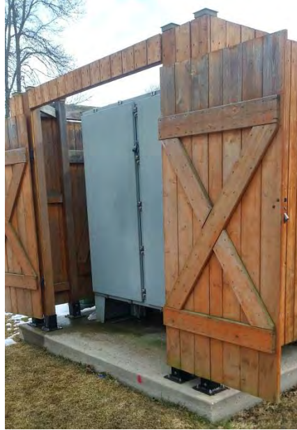
Figure 17 – Pumping Station No. 13 Utility Locker
