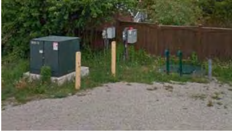
Figure 12 – Pumping Station No. 10 Image Source: Google Maps
