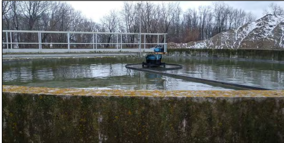
Figure 4 – Primary Clarification Ditch
