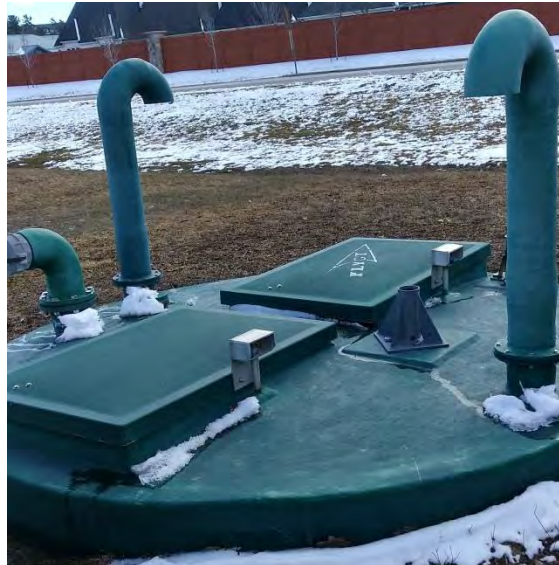
Figure 6 – Pumping Station No. 5
