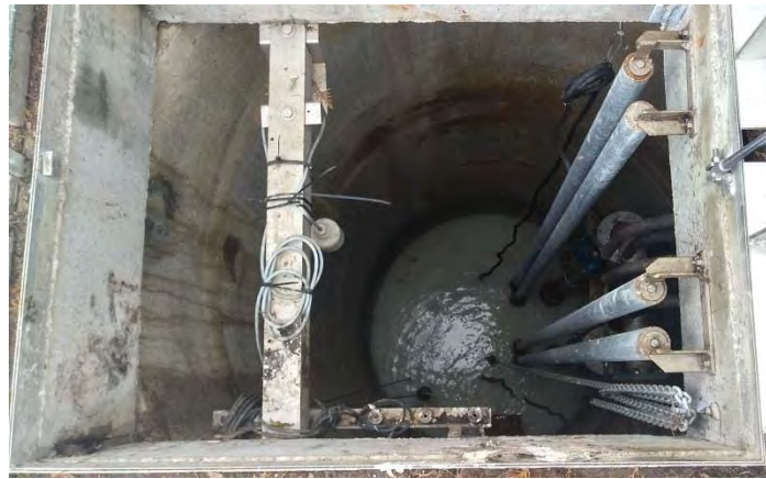
Figure 27 – Pumping Station No. 20
