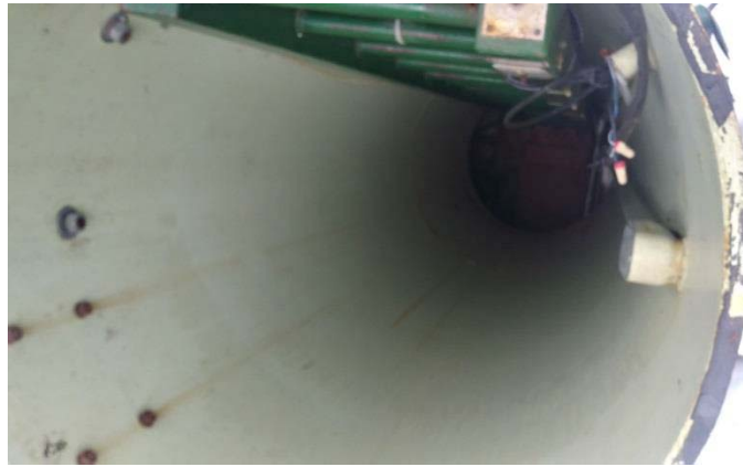
Figure 16 – Pumping Station No. 12 (Canister Station)
