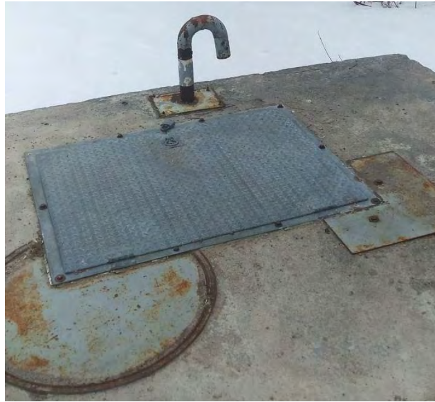
Figure 5 – Pumping Station No. 4
