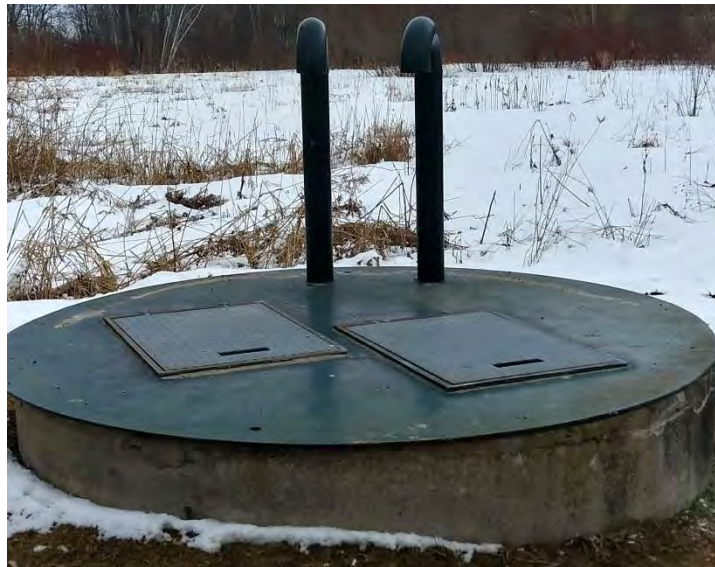
Figure 21 – Pumping Station No. 16
