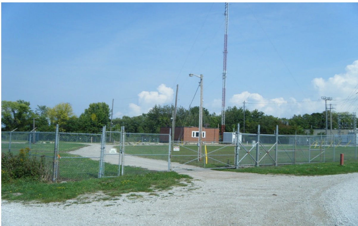
Photograph 1: View of radio tower and Hydro sub-station looking south
