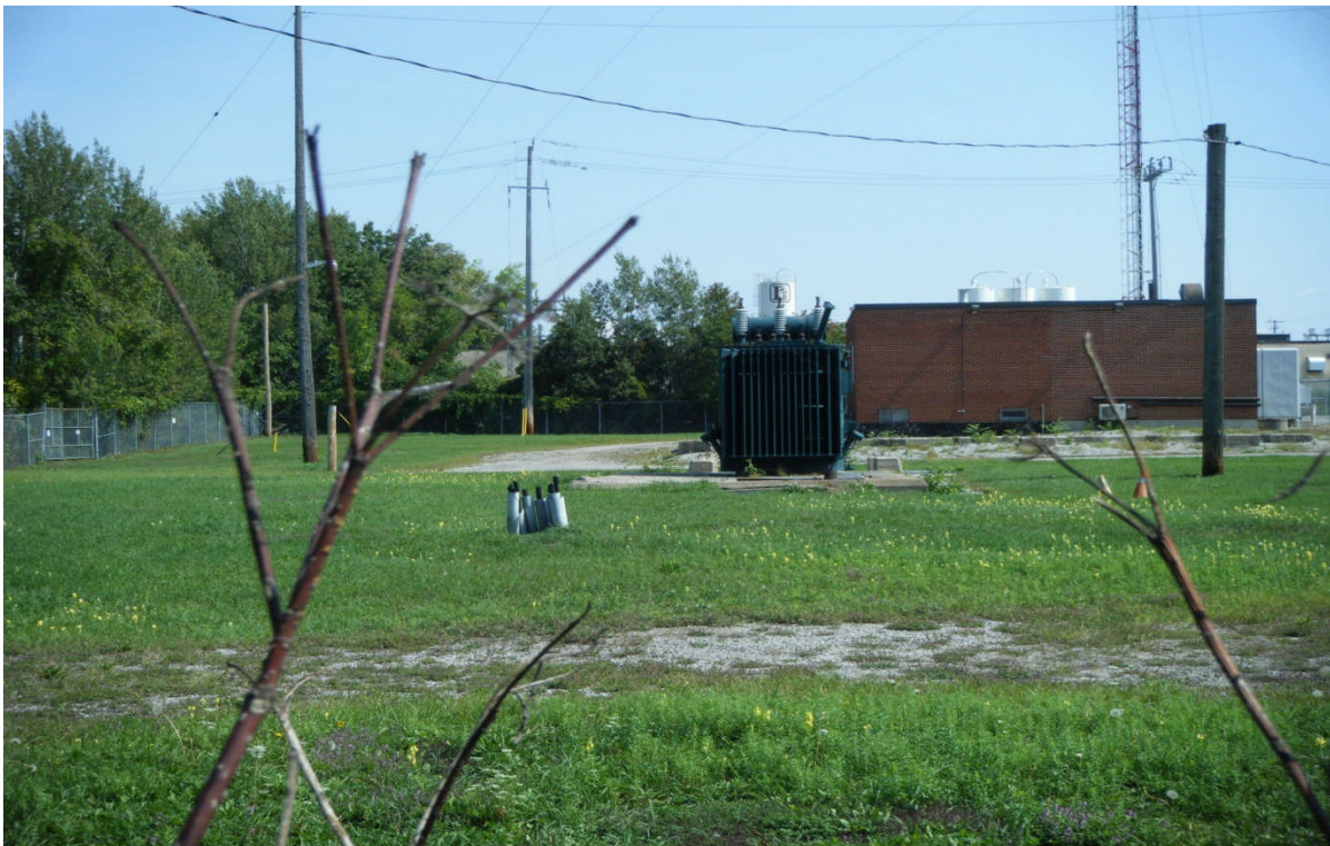
Photograph 6: Transformer located adjacent to the radio tower
