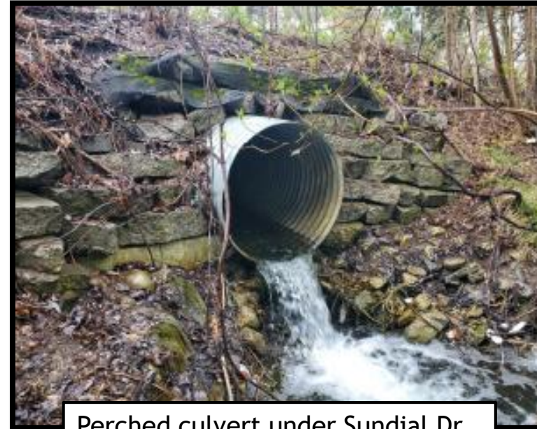
Perched culvert under Sundial Dr.
